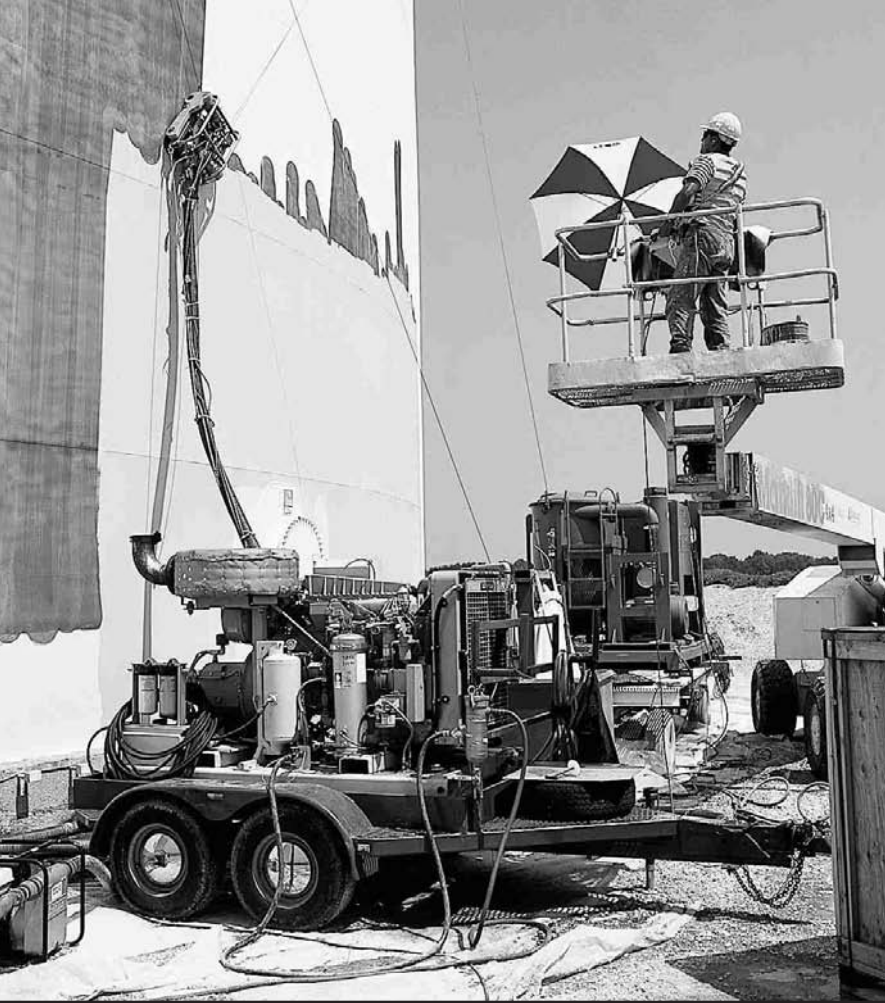
Shown above: HydroCat removing coating from the storage tank in excess of 500 square feet per hour. Surface prepared to NACE/SSPC WJ-1 or near white metal.
